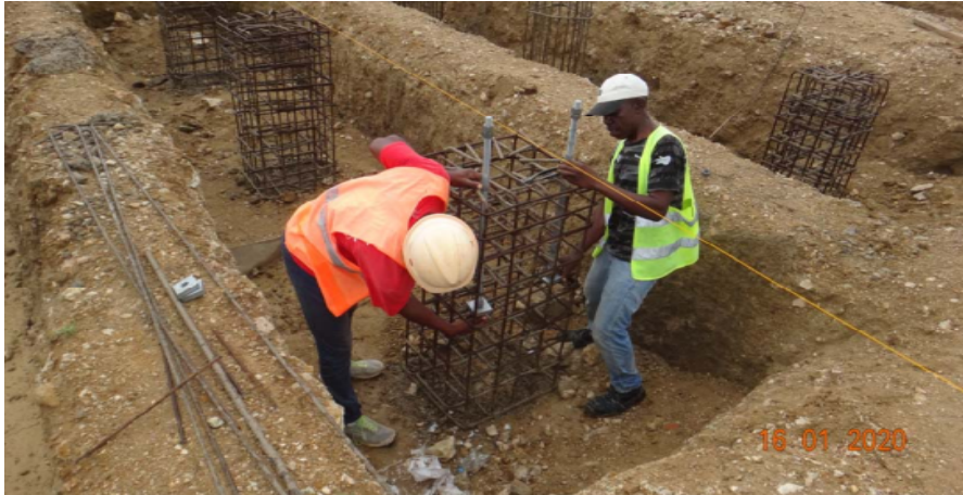
Photo 9-2: Staff are Contractors Staff are Fixing Bolts in Columns Without Wearing Groves to Protect their hands against injuries (Source: Progress report)
