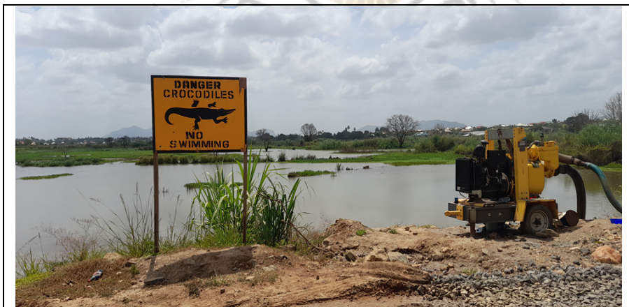
Photo5.2: The area affected by the ongoing construction of SGR. Photo taken 194km within Morogoro Municipality (Phot taken on 29 th January 2021)
